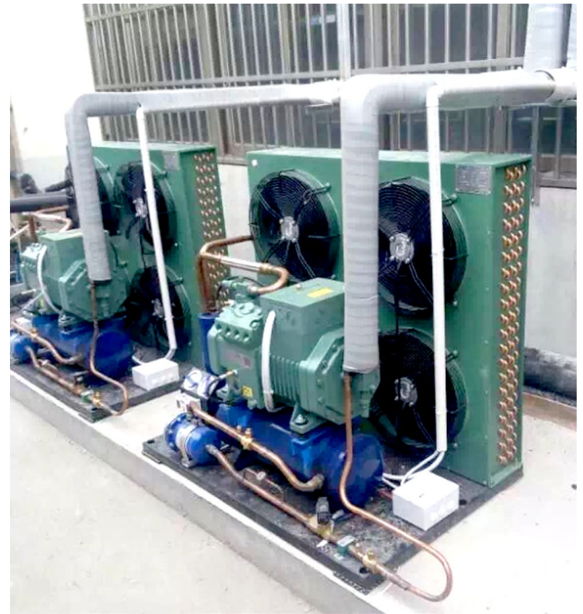
Figure 9. The compressor of application of the proposed research.
