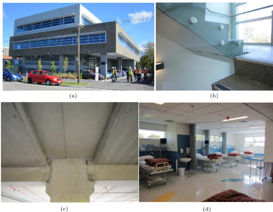
Figure 14. Precast hybrid structure [62]: (a) Exterior; (b) seismic damage; (c) frame; and (d) post-EQ operational.
