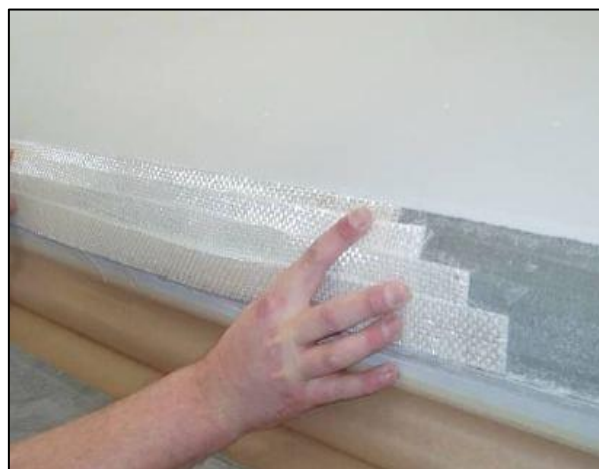
Figure 10 Application of glass filler in case of overbite repair that is leading edge offset
