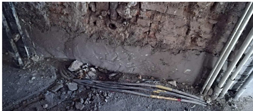
Figure 3. Wall and ceiling demolition for locating the Mechanical, Electrical, and Plumbing (MEP) installations.
